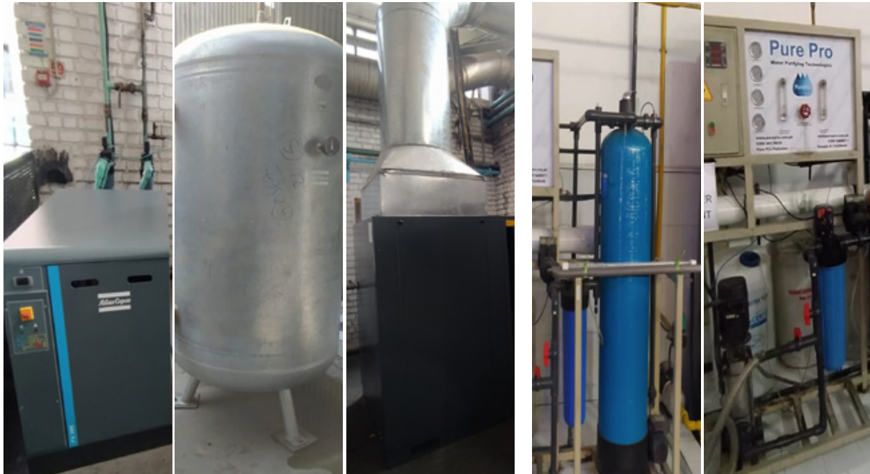
Atlas Copco Air Compressor Installation
